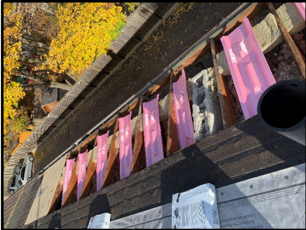
Provision of new preformed foam baffles between each rafter space at Units 4-8
