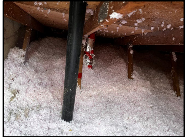
Provision and installation of new blown-in cellulose insulation within the attics of Units 4-8
