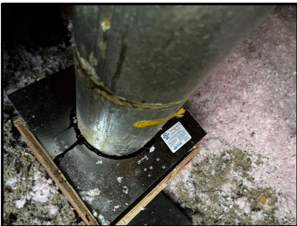
Locally seal penetrations in ceiling air/vapour barrier around b-vents & chimneys in attics of Units 4-8 with metal flashing and high temperature rated sealant
