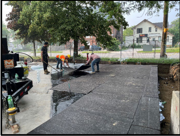
Provision of new waterproofing system at the garage roof slab at the north, east, and west sides of the building
