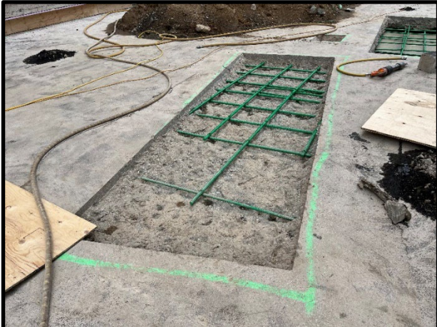
Localized concrete top surface repairs at the garage roof slab at the north, east, and west sides of the building
