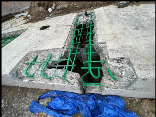
Localized concrete through slab repairs at the garage roof slab at the north, east, and west sides of the building
