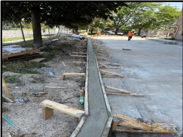
Provision of new concrete curbs along the paved areas at the north, east, and west sides of the building
