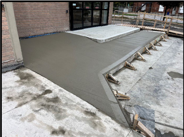
Removal and replacement of concrete walkways, entrance landing, and steps at the on-slab paved areas
