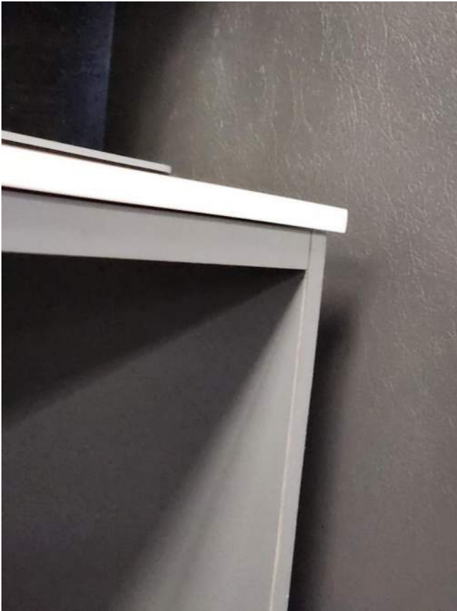
Figure 10 - Solid surface countertop edge detail does not appear to conform to kitchenette millwork drawing/detail.
