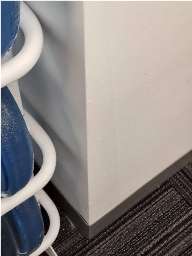
Figure 9 - Minor damage noticed at GWB wall corner edges.
