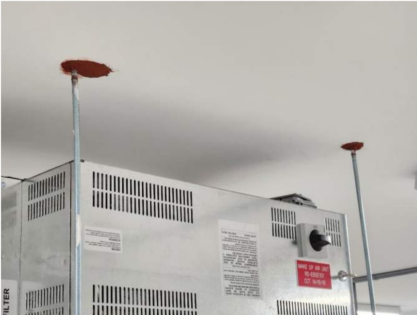
Figure 17 - Existing C.A.C.F. Room (EBS013) Ceiling mounted make-up air unit is missing fire-rating labels at threaded-rod ceiling penetrations.
