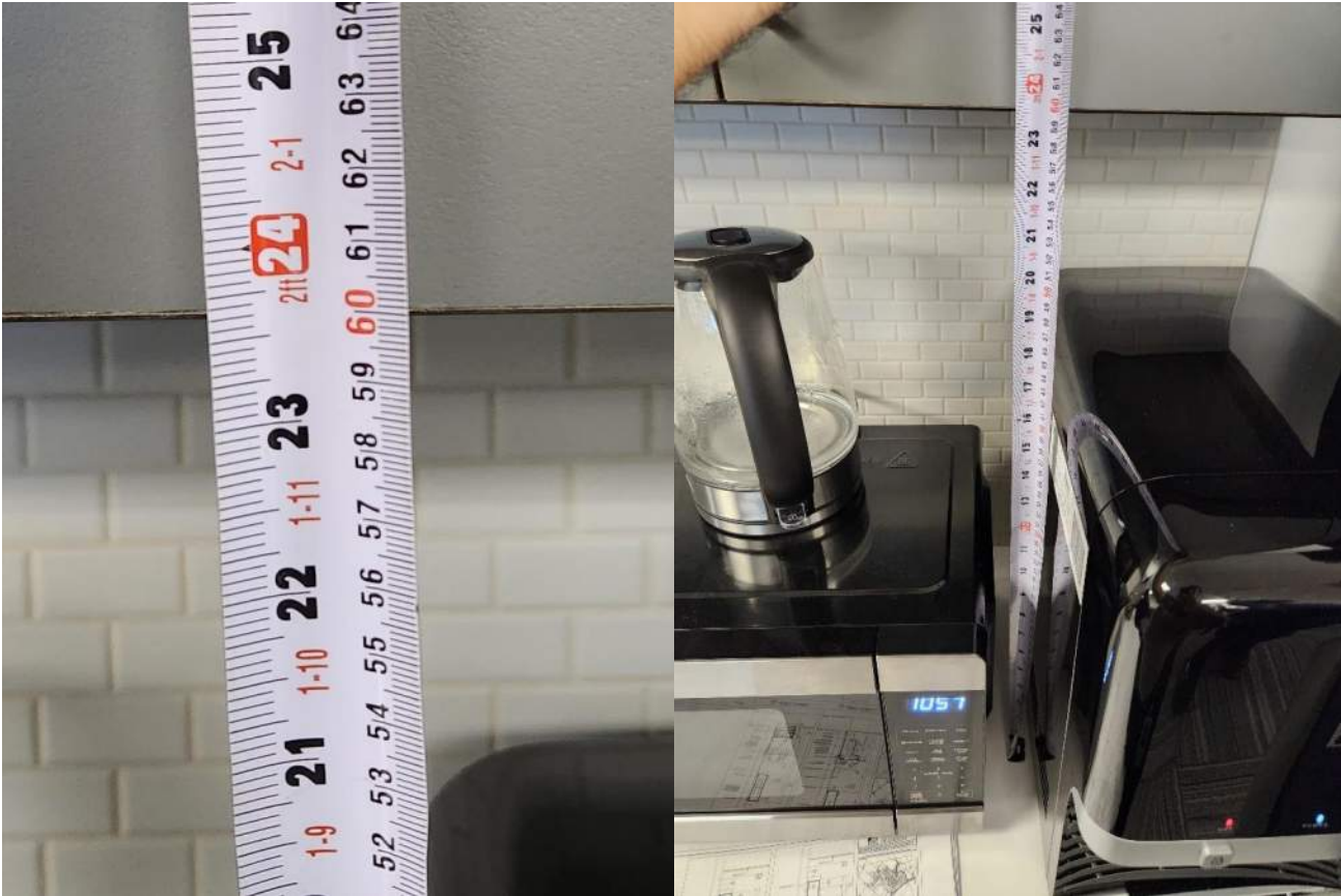
Figure 14 - Heigh of millwork cabinet uppers from countertop was measured at: 600 mm, drawing shows: 590 mm.
