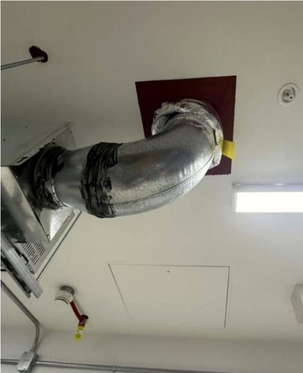
Figure 25 - Site Installation of MAU Ductwork Not Conforming to Manufacturer's Instructions
