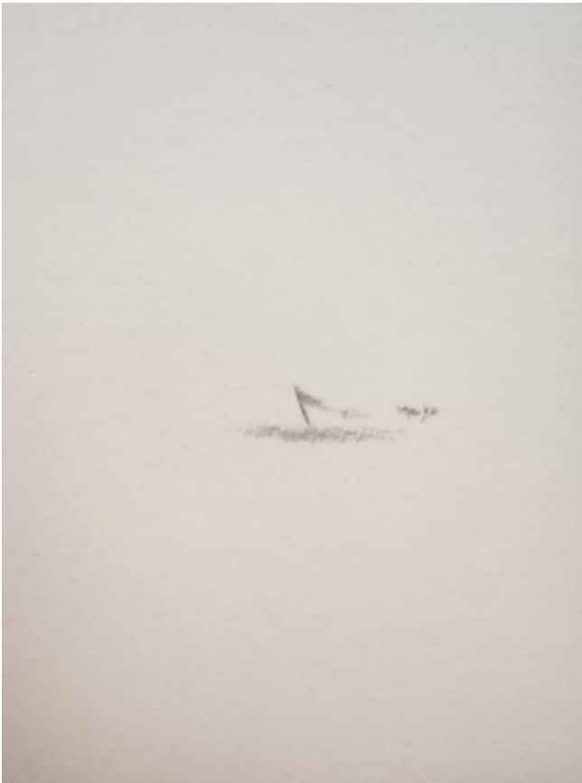
Figure 5 - Scuff marks / smudges on several walls.
