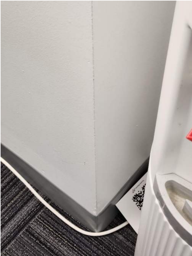
Figure 8 - Minor damage noticed at GWB wall corner edges.
