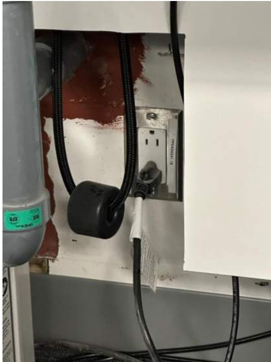
Figure 28 - Receptacle below sink in BMS Office EBS019
