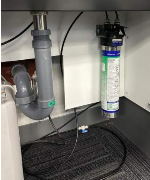
Figure 19 - Under-sink water filter.
