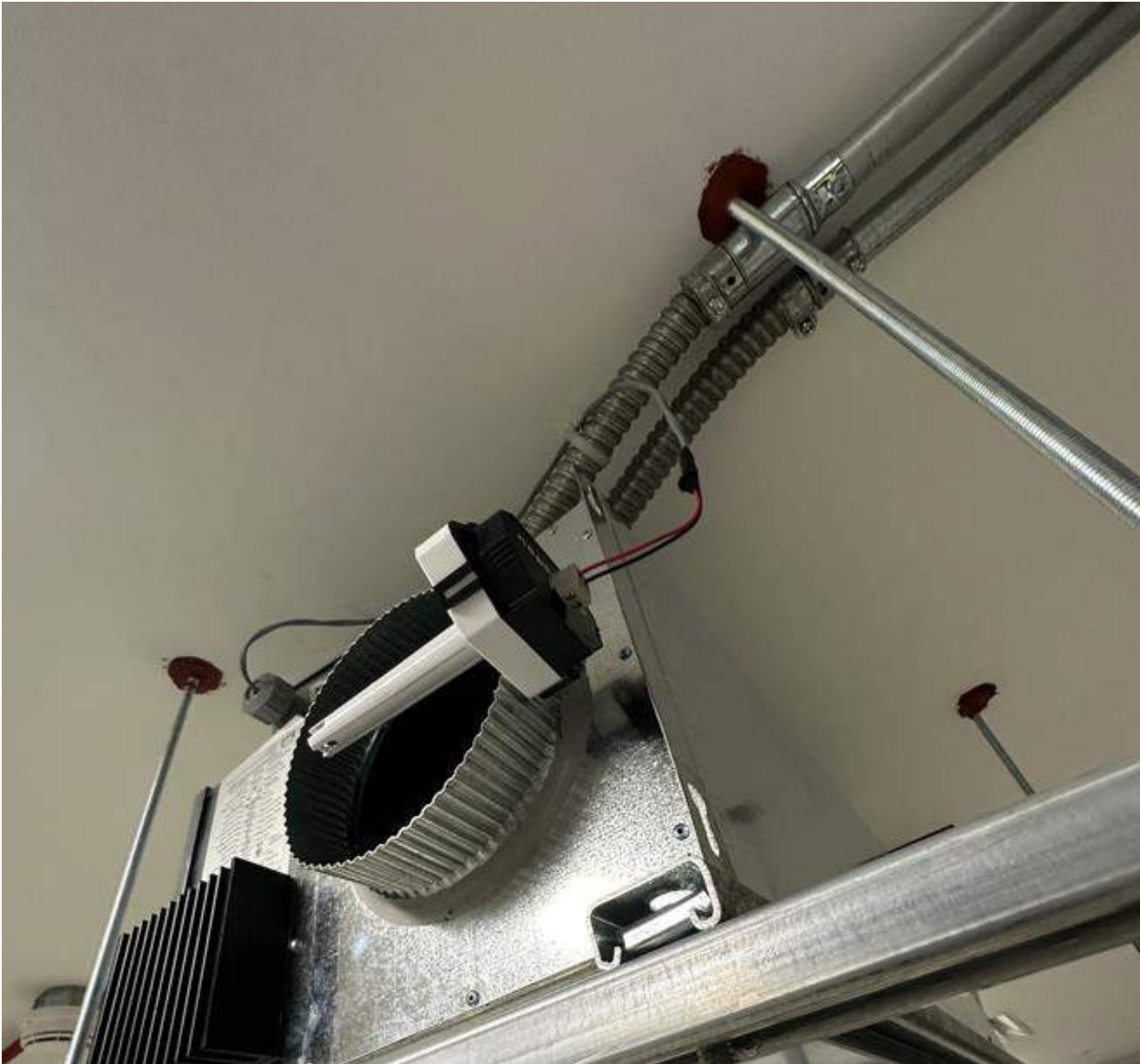
Figure 27: Thread rods do not have fire rating labels.
