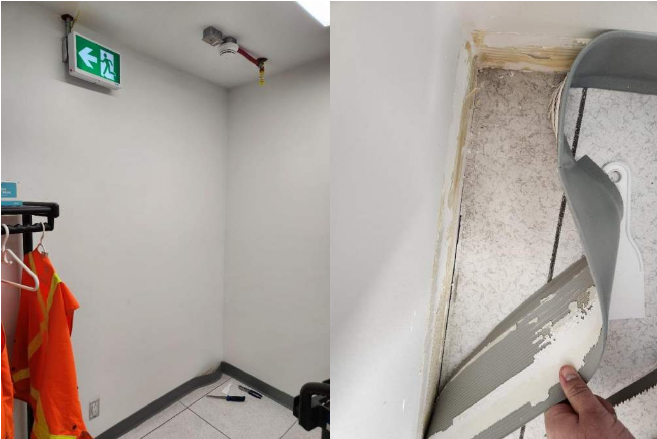
Figure 18 - Existing C.A.C.F. Room (EBS013) fire rated (red) caulking was not visible below fire rated GWB partition wall. Concern about installation of firestopping around new fire rated walls. This is to be verified as it is an occupant life-safety requirement according to the building code.
