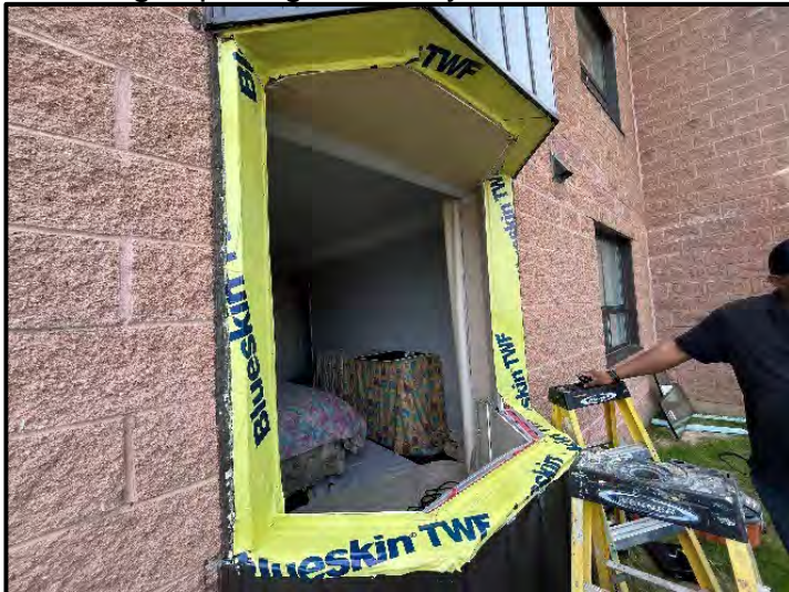
Installation of membrane flashing of the rough opening of the bay window at unit 108
