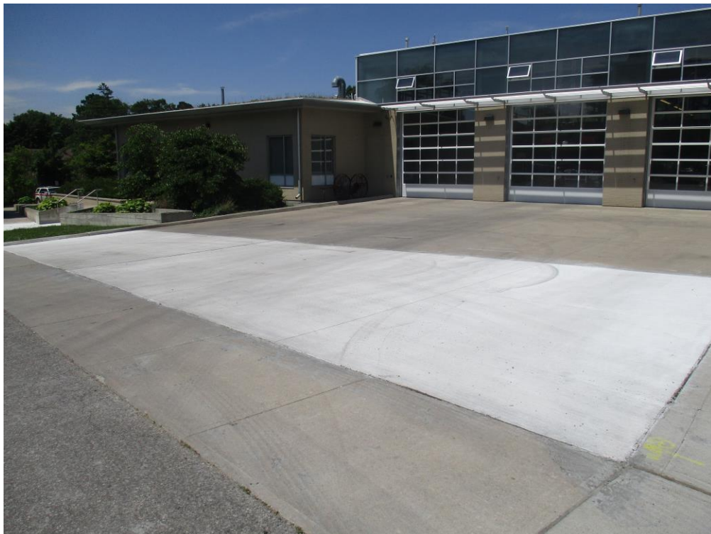
Photo 2: Interlock pavers and granular materials for area #3 has been removed and replaced with reinforced concrete slab.
