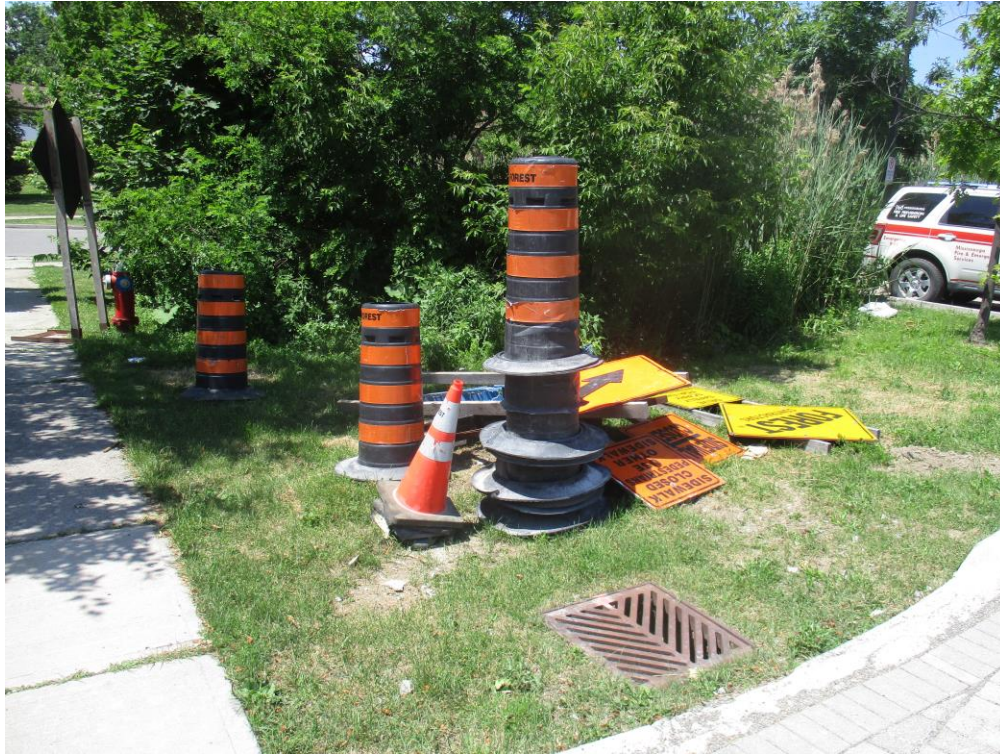
Photo 8: The contractor was instructed to remove all the signs and construction cones on the green zone area adjacent to area#2 and all areas disturbed by construction shall be restored to the original condition by providing local fill, a minimum 100mm topsoil and 50mm sod.
