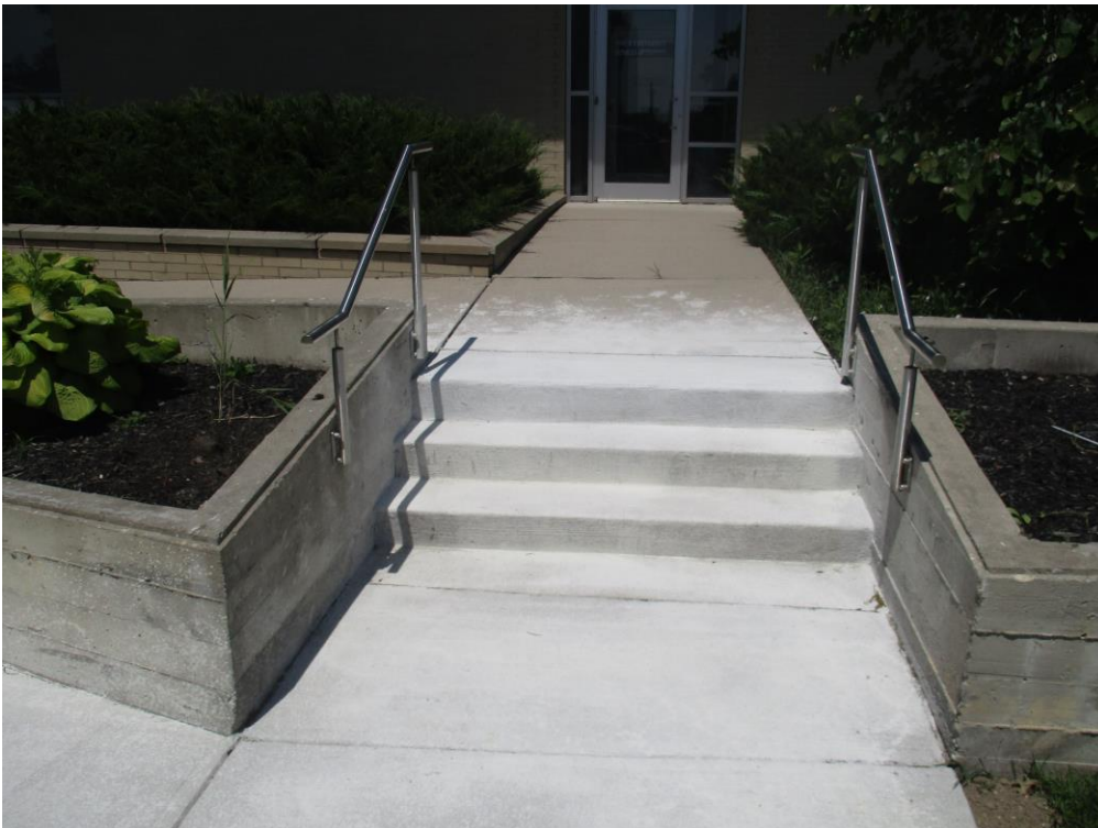
Photo 7: The contractor was informed to wash and clean adjacent the repaired concrete areas# 3 & 4 and send photo to our office for review and record after completion of work.
