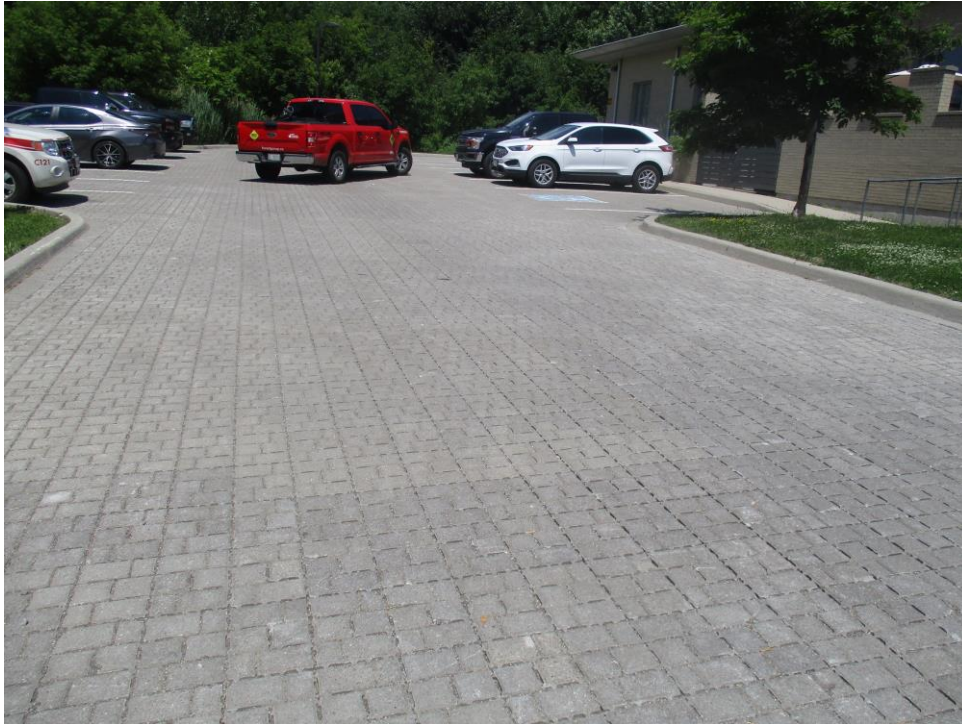
Photo 3: Interlock pavers and granular materials for areas#1 &2 have been removed, granular materials was replaced, compacted and interlock pavers have been reinstated.
