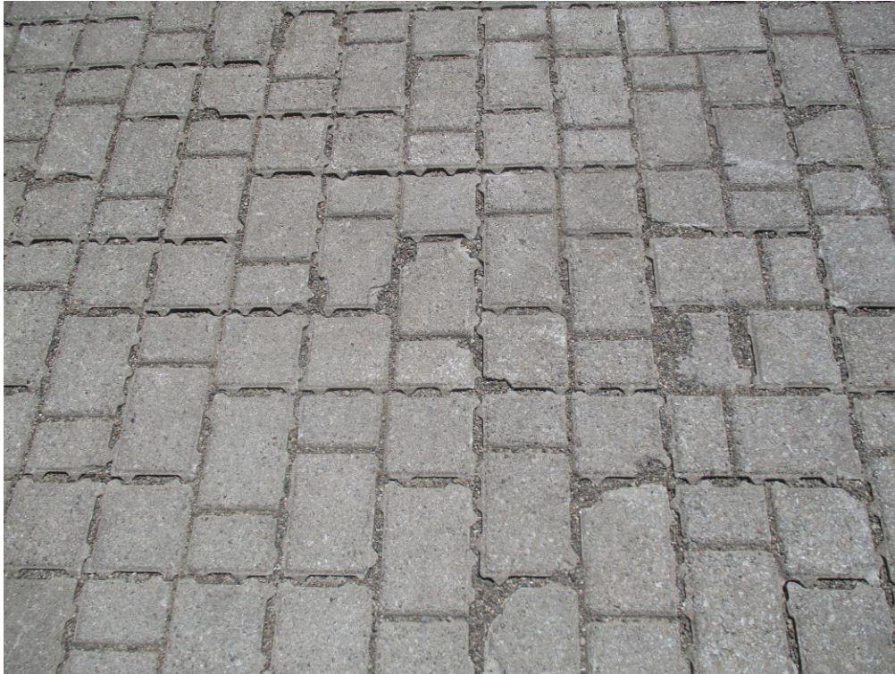
Photo 5: Chipped interlock pavers for areas# 1 & 2 are to be replaced with new interlock pavers as per the contract document, the contractor was instructed to send photo to our office for review and record after completion of work.
