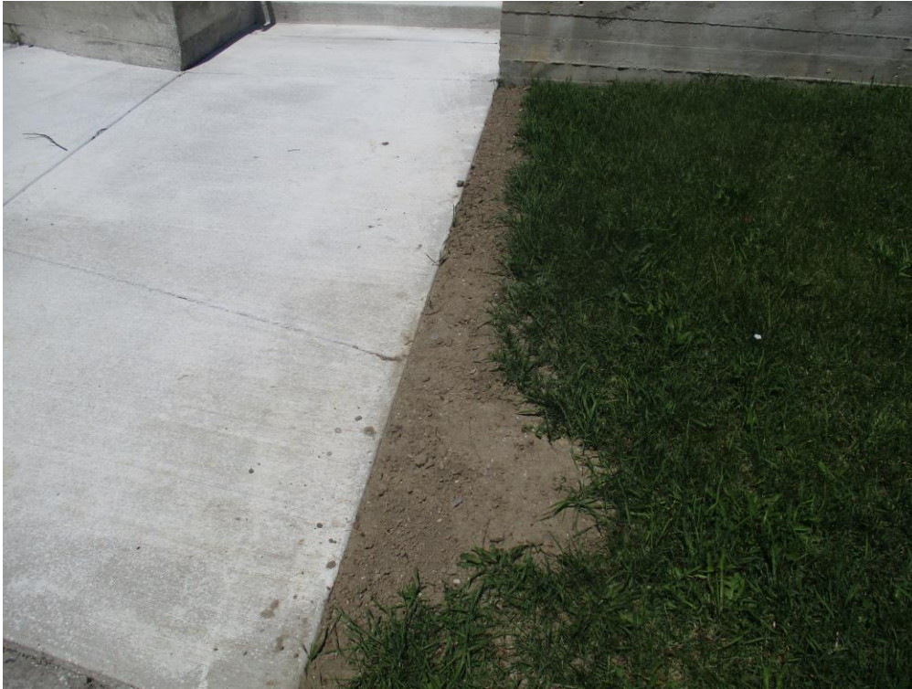
Photo 6: All areas disturbed by construction and adjacent concrete sidewalk shall be restored to the original condition by providing local fill, a minimum 100mm topsoil and 50mm sod, the contractor was advised to send photos to our office for review and record after completion of work.
